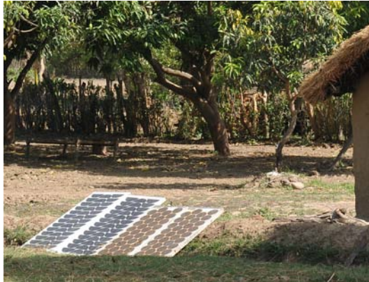
Figure 2.6.: Solar panels on the edge
